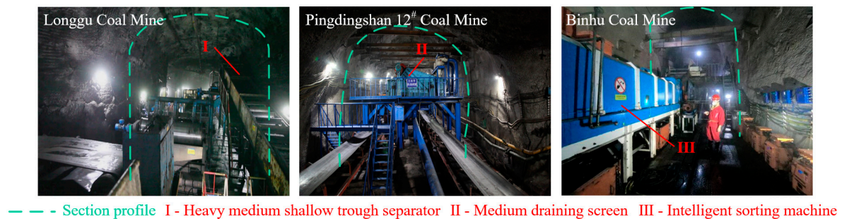
Figure 2. Underground chamber for coal–gangue separation.
