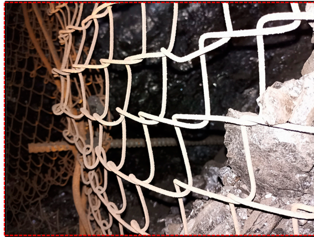
Figure 3. Coal mass on roadway rib bulge outward and severe damage to the support system.
