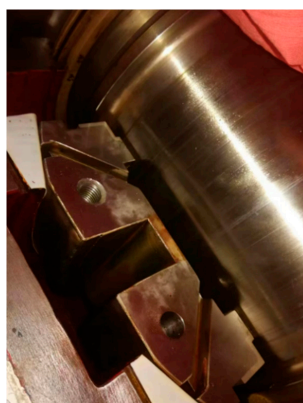
High temperature of bearing (H2)
