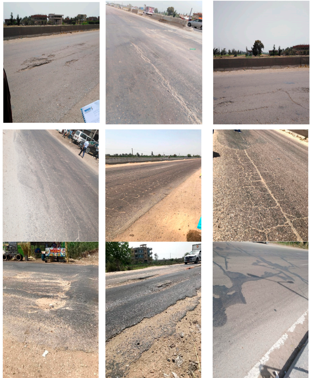
Figure 4. Surface distress of pavement based on visual inspection.
