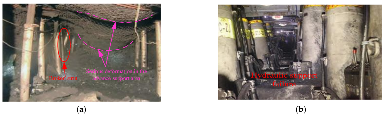
Figure 1. Site strong mineral pressure appears. (a) Over-supported monolithic column fracture. (b) The hydraulic support at the working face is crushed.
