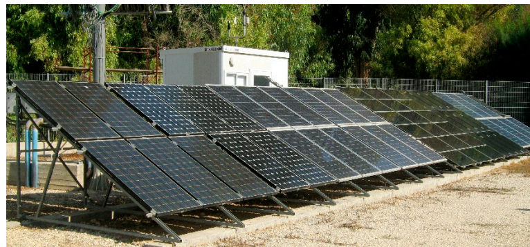
Figure 1. PV arrays installed at the UCY in Nicosia, Cyprus.
