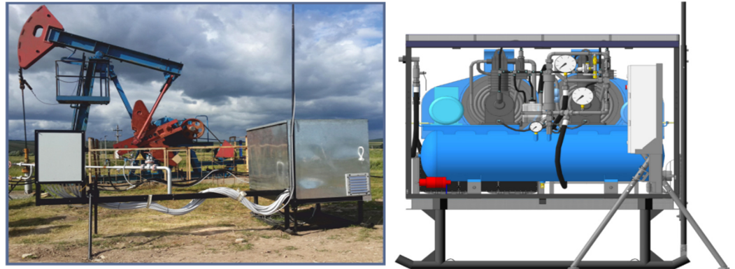
Figure 1. A set of equipment for gas extraction from wells (KOGS).
