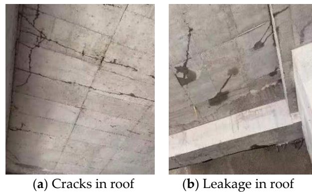
Figure 1. Photograph of the cracked concrete structure in a metro station in Xi'an China.
