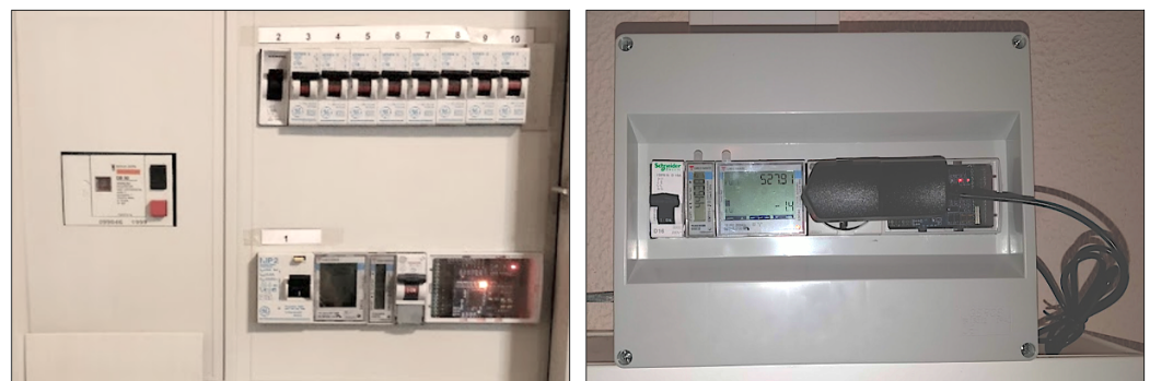
Figure 2. Example of two installation from the case study. On the site at left all the equipment was installed in the site main breaker box. The picture at right depicts another site in which all the installed equipment had to be installed in a adjunct box.
