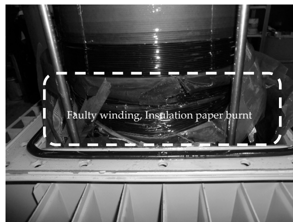
Figure 12. Pictorial description of the location of failure in the set-3 distribution transformer suffering thermal fault: Insulation damage, winding burnt.
