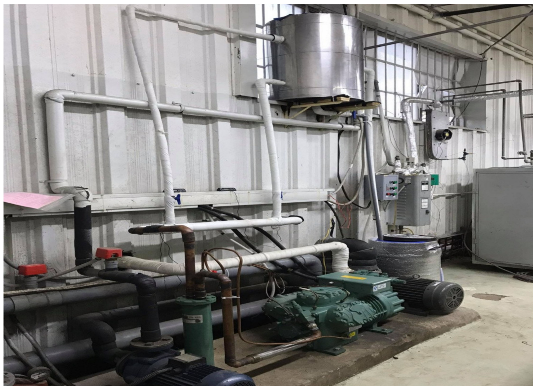
Figure 7. Photograph of the thermal storage tank integrated into the system.
