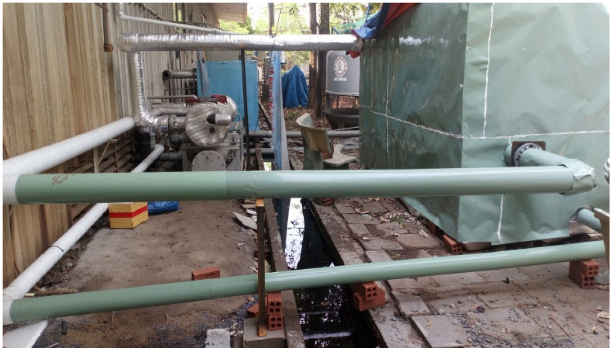
Figure 5. Photograph of the cold storage tank integrated into the system.
