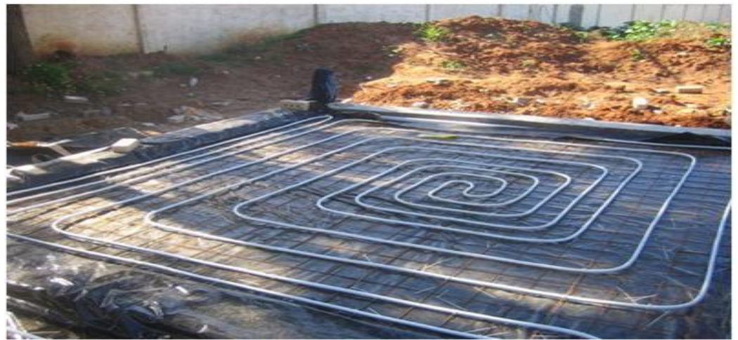
Figure 3. Floor piping presentation in Zone 1 (living room).
