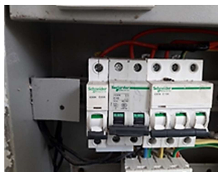
Figure 7. Fire alarm fault detected and repaired at circuit breaker level.
