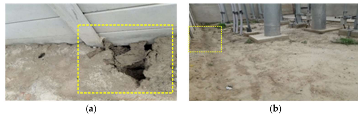
Figure 6. (a) Boundary wall support soil displaced due to rain, and (b) boundary wall support soil rectified.
