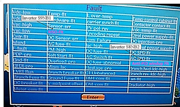
Figure 4. Inverter faults as seen on the SCADA screen.
