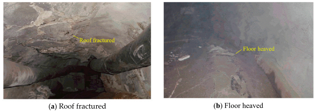
Figure 4. Roadway failure characteristics under the initial supporting design.
