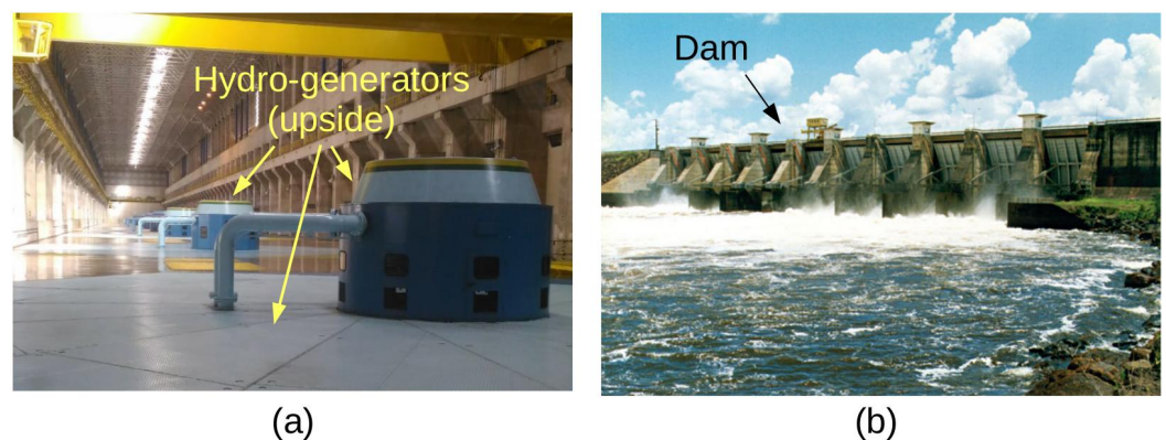
Figure 2. Hydro-electric power plants involved in this study: (a) Generator hall of Tucuruí power plant; and (b) outside view of Coaracy Nunes power plant.
