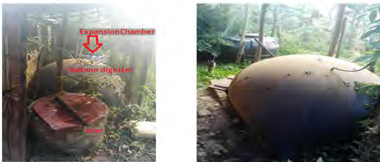
Figure 7. Balloon type digester.
