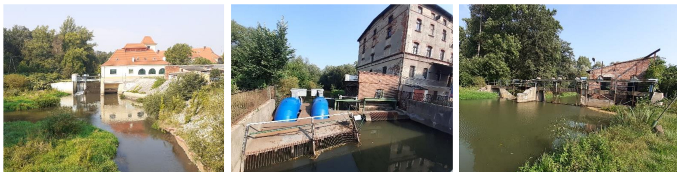
Figure 2. Research facilities (from left): Marszowice, Skalka, and Sadowice hydropower plants.
