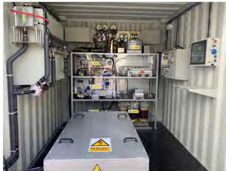
Figure 5. DC/AC converter for conversion converting trolleybus 600 V DC overhead line voltage into a 400 V AC commercial standard (operating in Gdynia, Poland; the battery-based energy storage is in the box placed on the floor).
