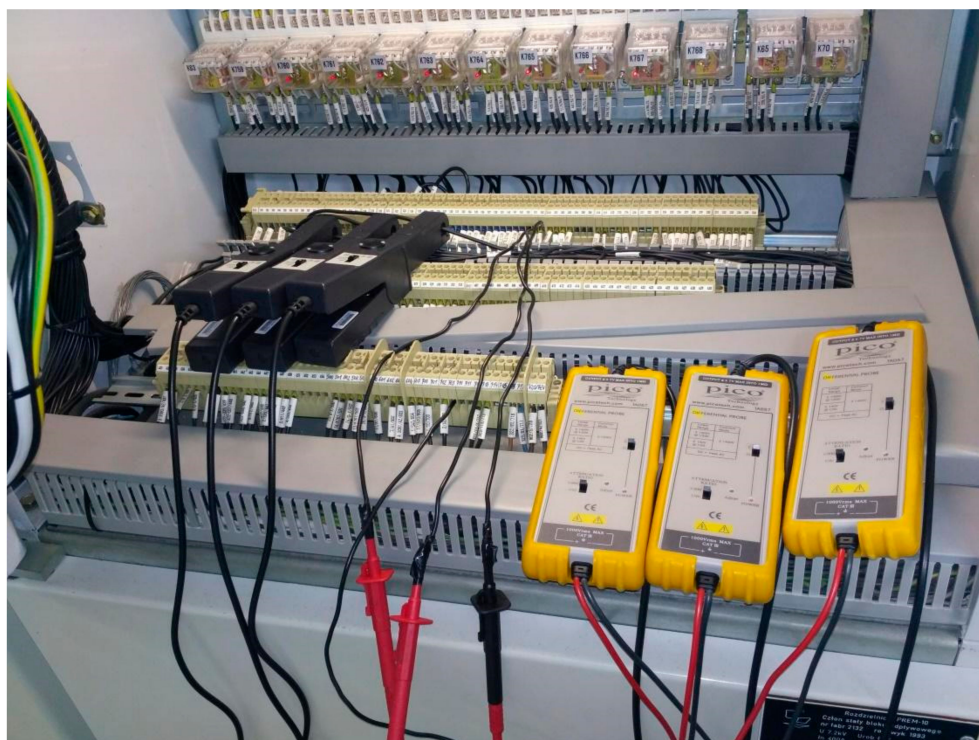
Figure 17. Current and voltage probes clamped on protection circuits in the switchroom.
