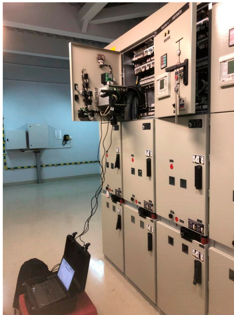
Figure 16. Measurement of current signals from secondary circuits in the switchroom.
