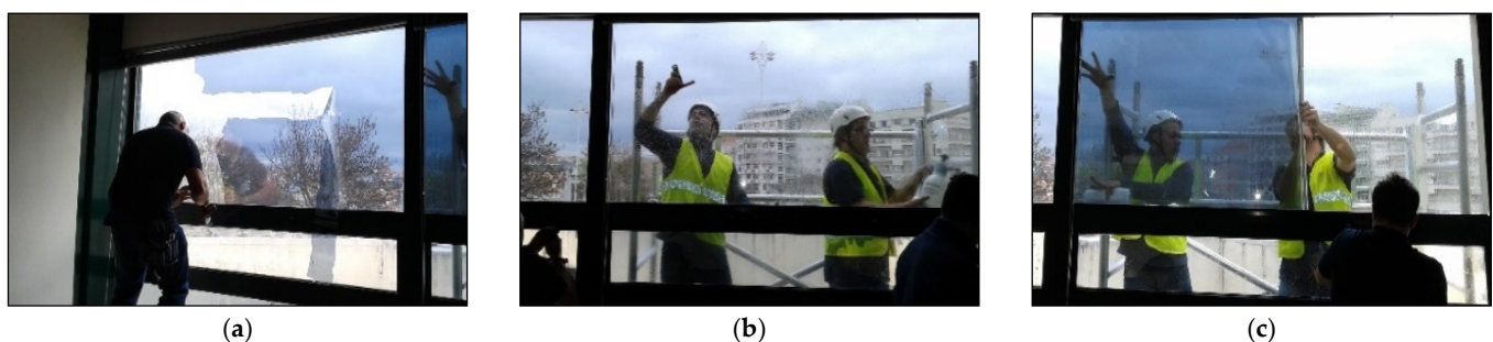
Figure 4. Internal view of the removal of the existent solar control film (SCF) and installation of the new SCF in office I: (a) removal of the existing SCF B (internally applied on the glazing); (b) cleaning works of the external glass surface of the glazing; (c) installation of SCF A on the glazing (external glass surface).
