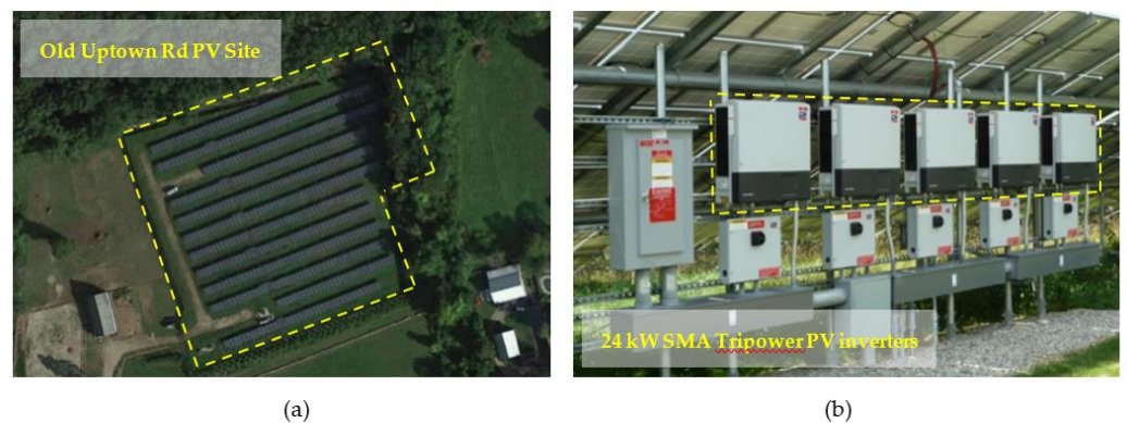
Figure 10. Field Demonstration. (a) Aerial View of the Old Upton Rd PV Site. (b) PV Inverters at the PV Site.
