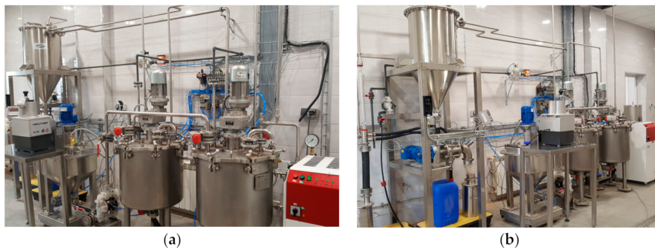
Figure 4. Photographs of an installation located in the sugar factory at Dobrzelin for processing beet pulp and beet leaves into furfural on a quarter-technical scale (a) right side view (b) left side view.
