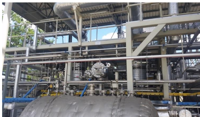
Figure 6. Photo of a fragment of the liquefaction system of post-cracking products and one of the intermediate tanks.
