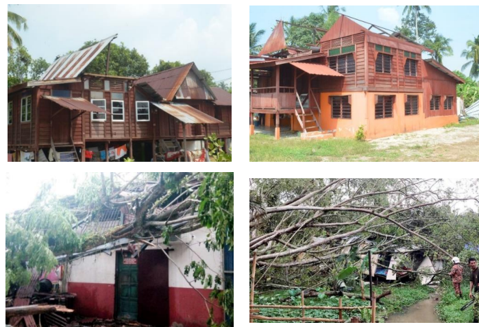
Figure 1. Tropical cyclones damage in rural areas in Malaysia.
