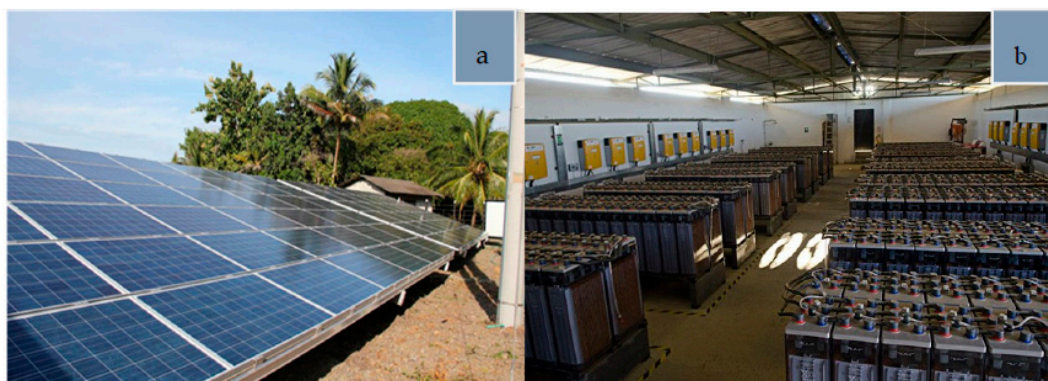
Figure 2. Current status of microgrids: (a) Titumate, and (b) Puerto Estrella.
