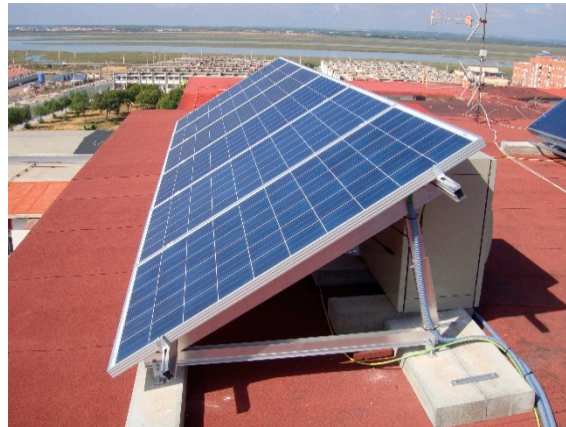
Figure 2. Several photovoltaic (PV) arrays on the roof.
