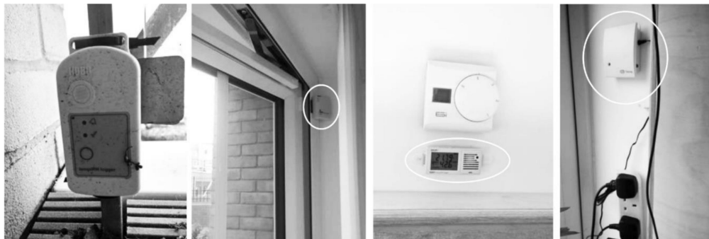
Figure 4. Environmental monitoring devices installed in the flats. From left: Outdoor temperature and RH logger, window state logger, interior temperature and RH logger and CO 2 loggers.
