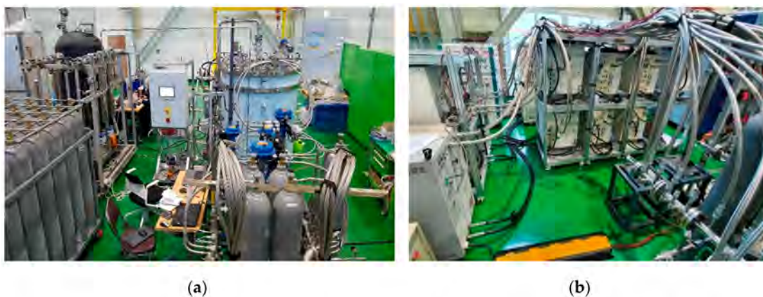
Figure 4. The constructed reverse Brayton cryogenic system: (a) cold box and pressure regulating system (PRS) and (b) compressor package.
