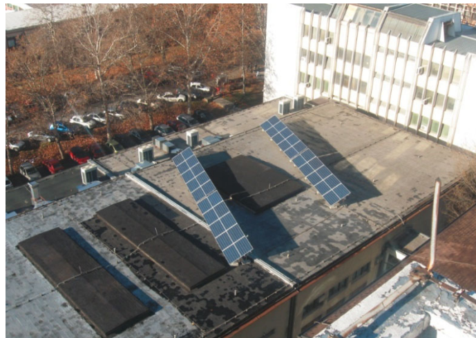
Figure 1. The overview of the PV power plant arrays from the FTS tower.
