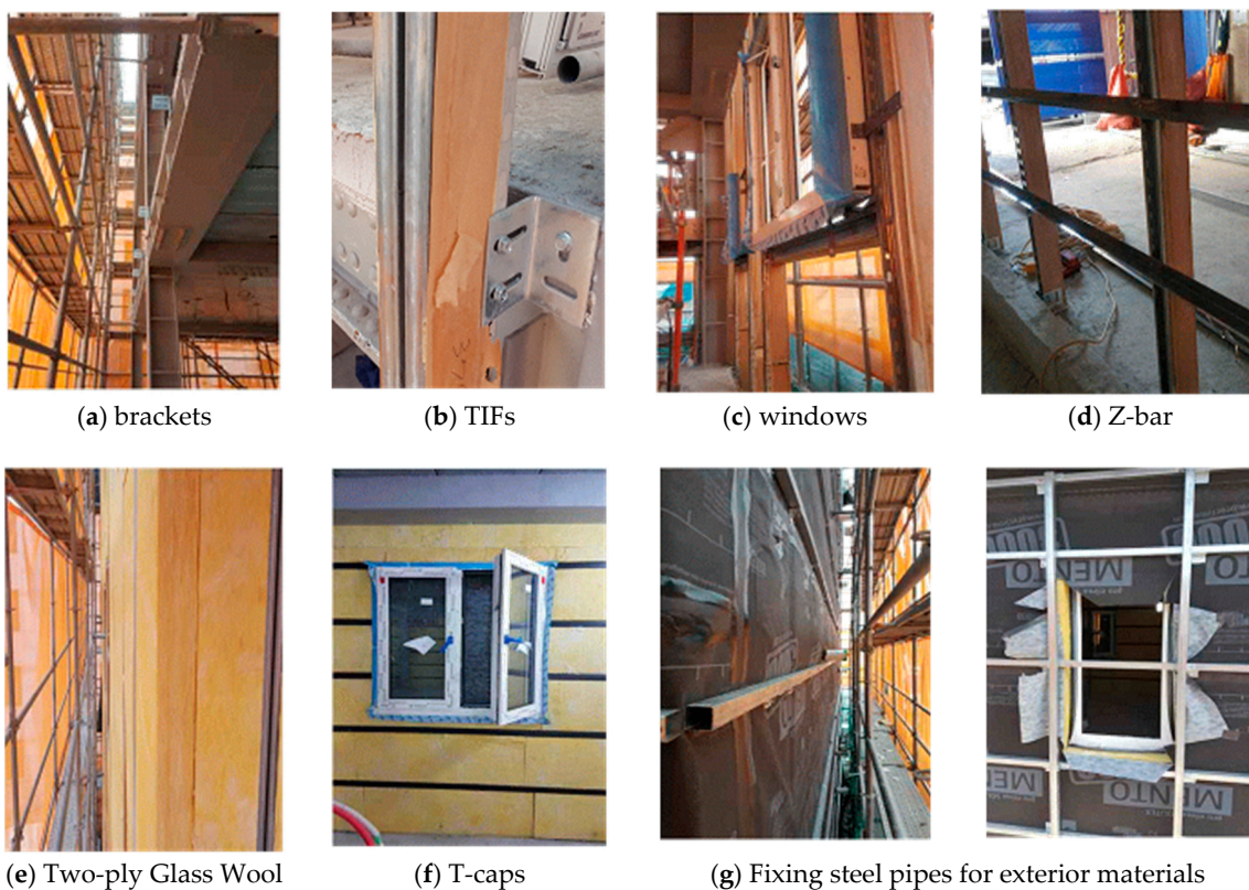
Figure 3. Construction of the TIF exterior insulation system on the curtain wall building.
