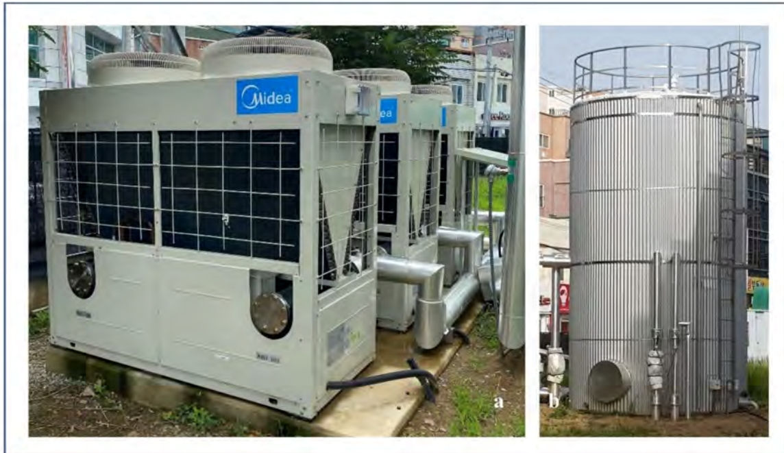
Figure 4. Field picture of (a) AWHP and (b) water storage tank.
