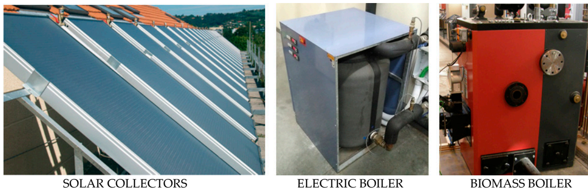
Figure 4. Heat supply sources installed in the GSCL.
