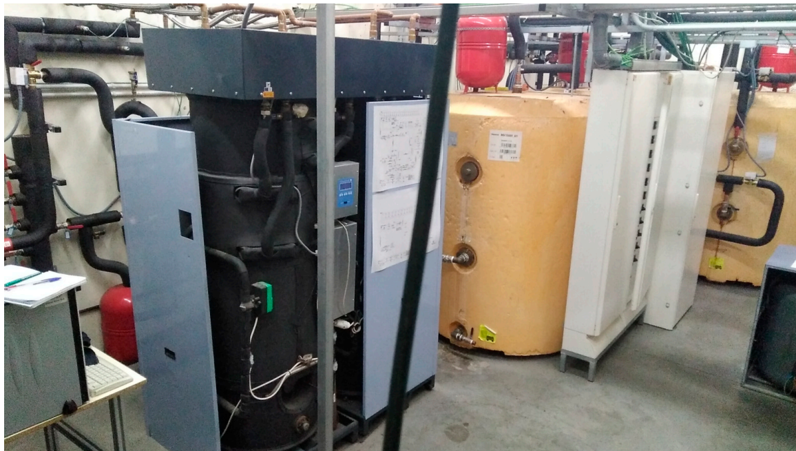
Figure 3. ClimateWell CW10 absorption machine installed in the GSCL.
