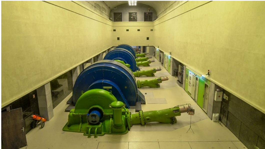
Figure 2. A view at the hydro power-plant turbine room.
