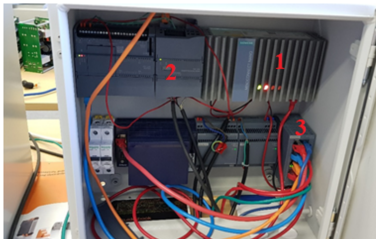
Figure 2. Data acquisition devices.
