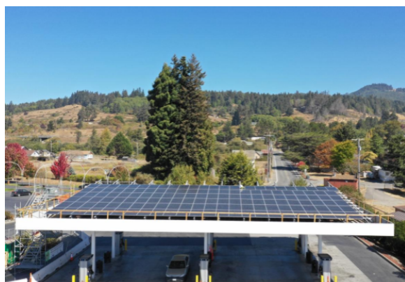
(a) 60 kW local solar power capacity
