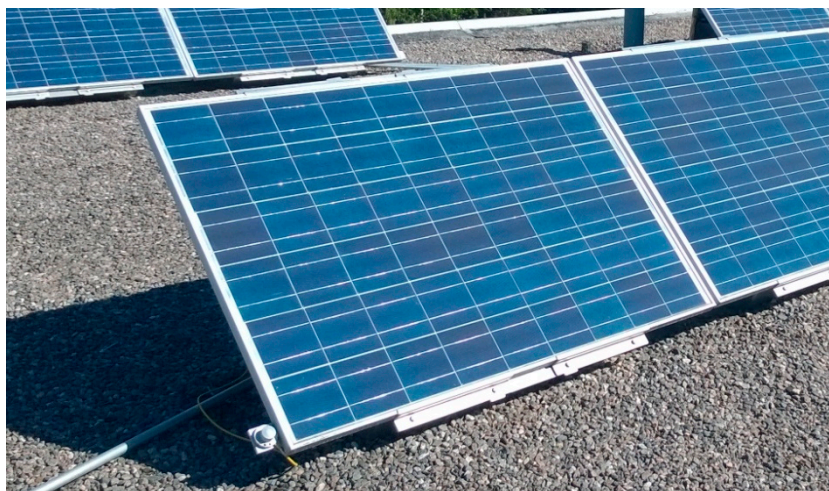
Figure 2. PV panel mounting and the pyranometer.
