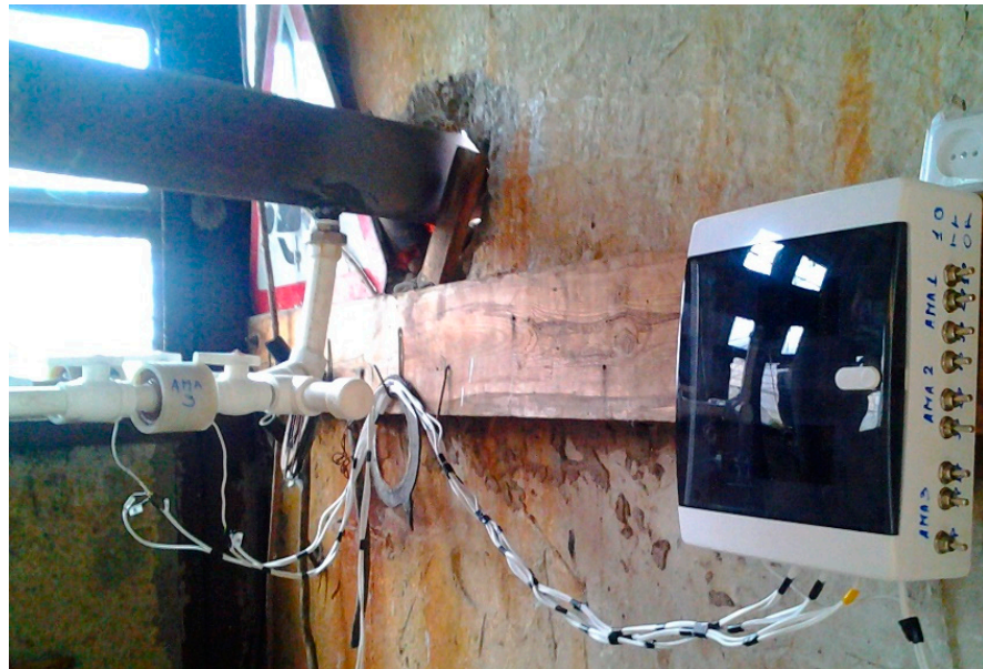
Figure 18. An acoustic–magnetic device with an automation system mounted on a geothermal supply pipe.
