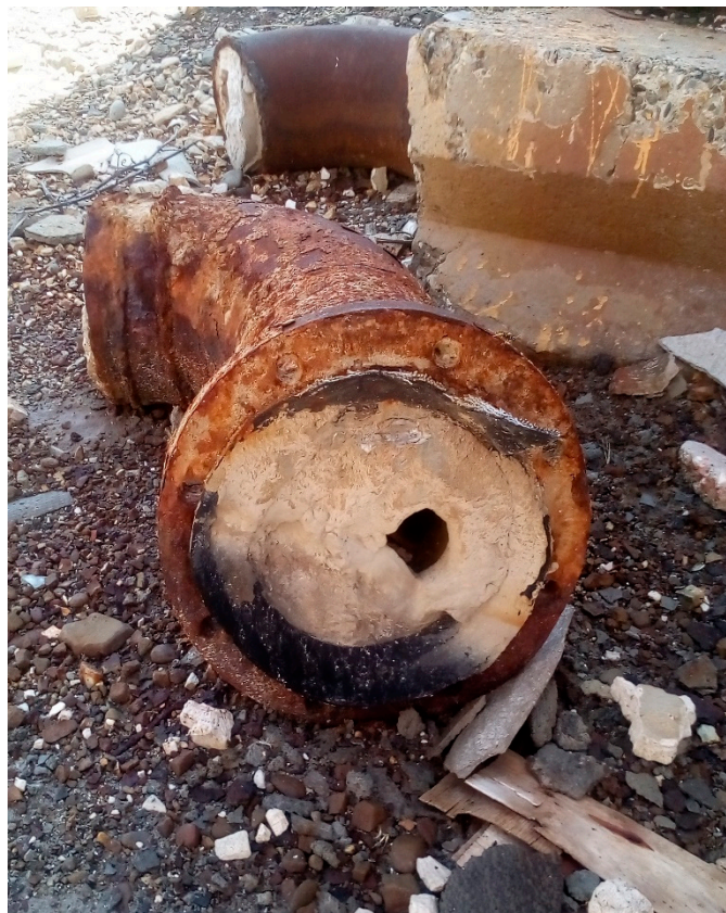
Figure 20. The appearance of a pipe in a geothermal heating system without an acoustic–magnetic device.
