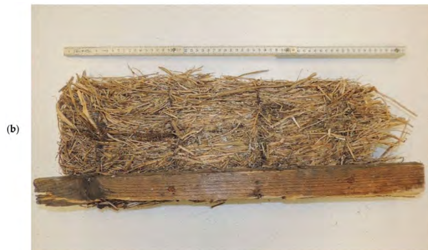
Figure 4. The finding condition of the SOLOMIT panel sample: (a) outer side, below, and (b) inner side with part of the fastening lath.
