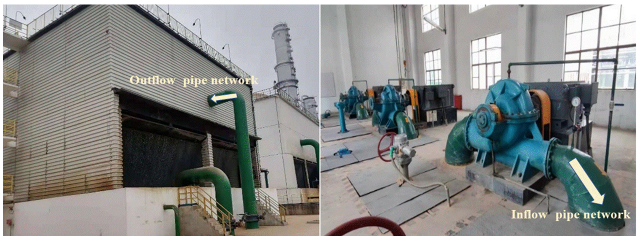
Figure 4. Cooling tower and water pump of the research object.
