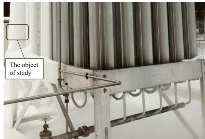
Figure 2. Finned tubes of LNG ambient air vaporizer totally covered by frost.
