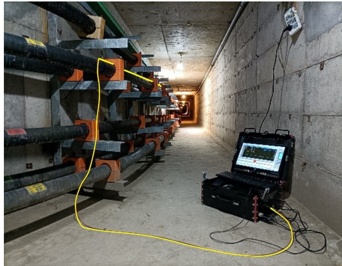
Figure 8. The cable temperature monitoring site.
