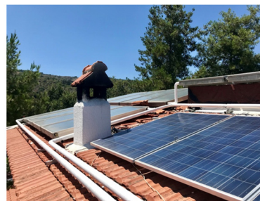
Figure 4. Solar collectors on the roof.
