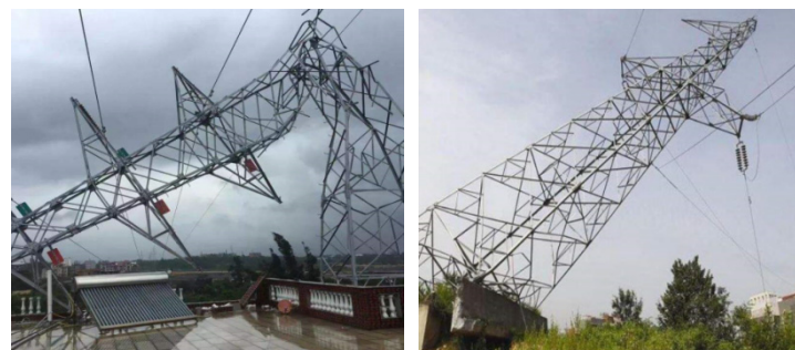
Figure 1. Tower collapse in typhoon weather.
