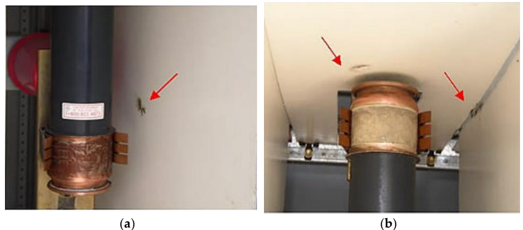
Figure 11. (a,b) show between a-phase and b-phase fuses; carbon trails may be seen on the insulation [36].
