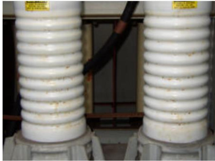
Figure 10. Contamination on ceramic bushing is caused by corona discharge [36].
