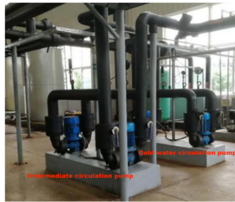
(b) Intermediate water and cold water circulation pumps
