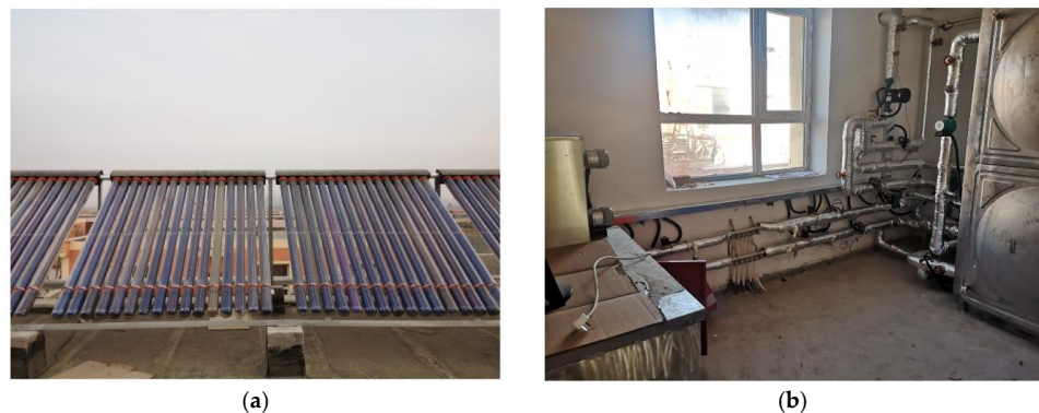
Figure 2. Equipment constituting MECH system: (a) VTC and (b) system pipeline.
