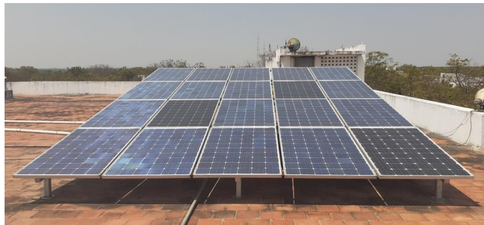
Figure 4. 5 kW PV Array.
