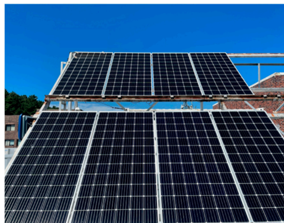
Figure 2. Photovoltaic system overview.
