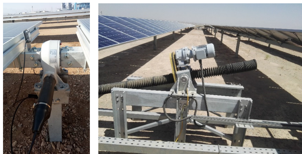
Figure 12. Two types of solar trackers installed in the Iranian power plants.
