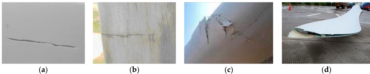
Figure 1. Typical images of defects: (a) scratch; (b) crack; (c) excoriation; (d) a blade cracked by lightning.
